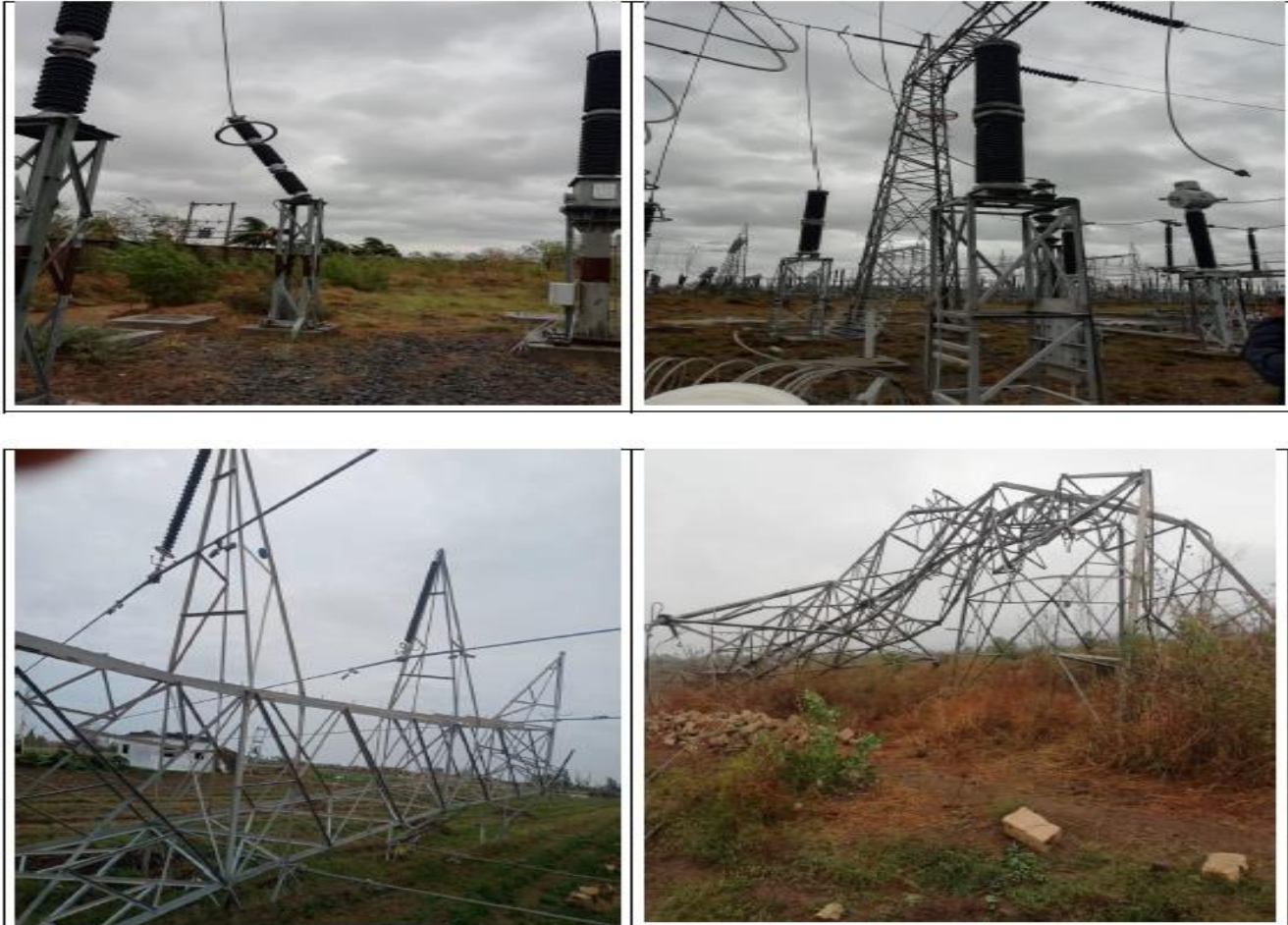
Photograph of Damages
